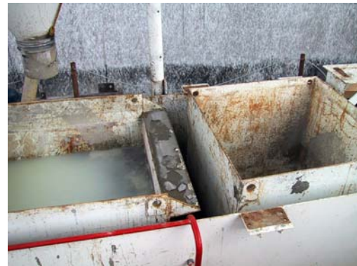
Slurry Cleaning Tank with Desander.
