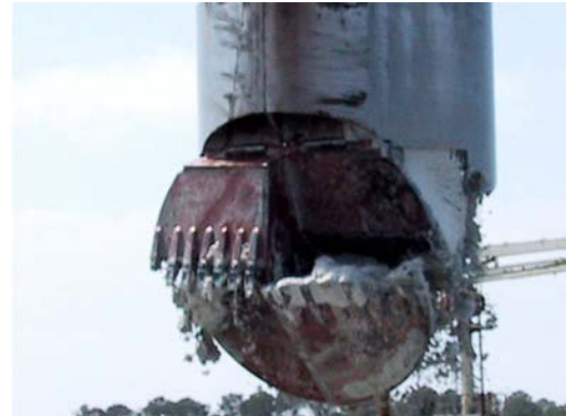
Digging Bucket used for loose sands and oyster shells. (click image to enlarge)
