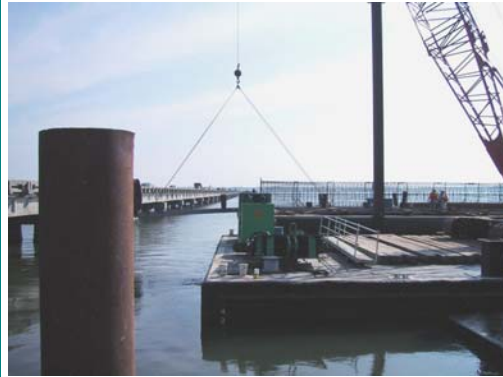
View of the old bridge & the rebar cage that is inserted into the drilled shaft prior to pouring concrete. (click image to enlarge)
