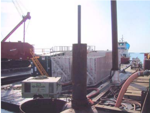
Slurry tanks on the barge next to the drilling barge. These tanks hold recycled slurry and fresh mixed batches of Shore Pac slurry. (click image to enlarge)
